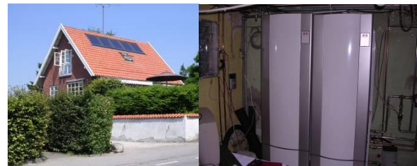
Left: Demonstration house with the solar heating system. Right: Solar tank and technical unit.
