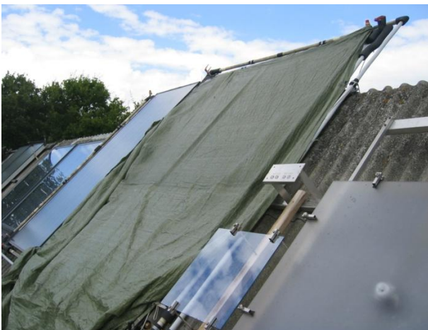
Fig. 3: Collectors with only one collector in use.
