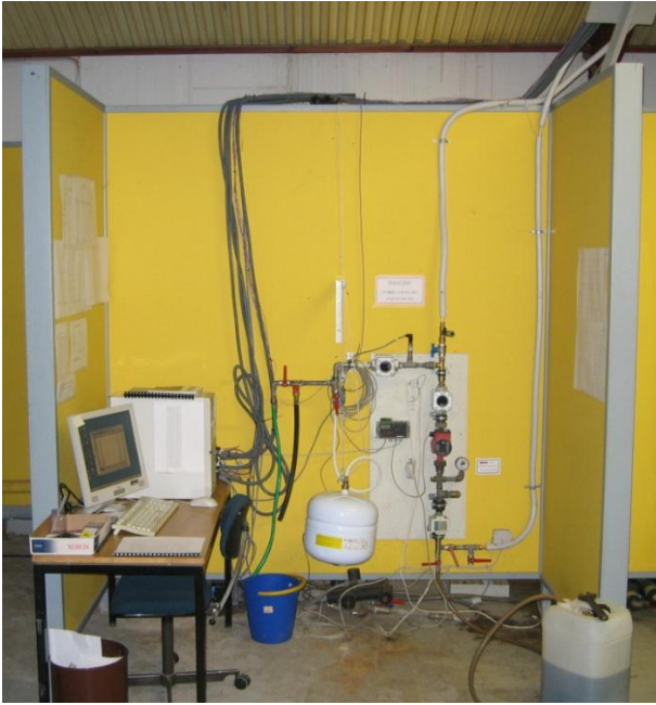
Fig. 2: System installed at BYG DTU.
