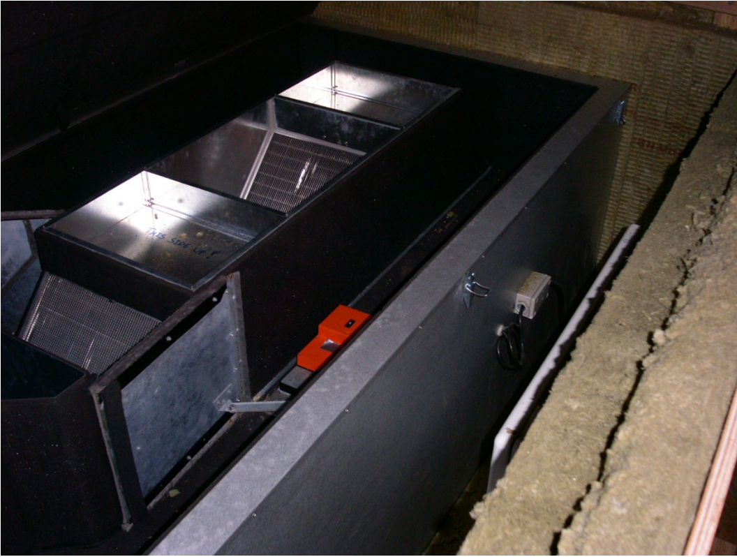
Figure 33 Heat exchanger in insulated box
