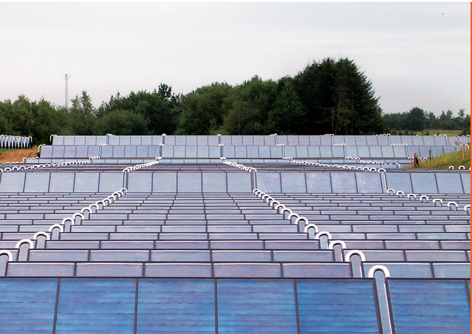
8000 m 2 solar collector field in Brødstrup. Photo: Jianhua Fan
