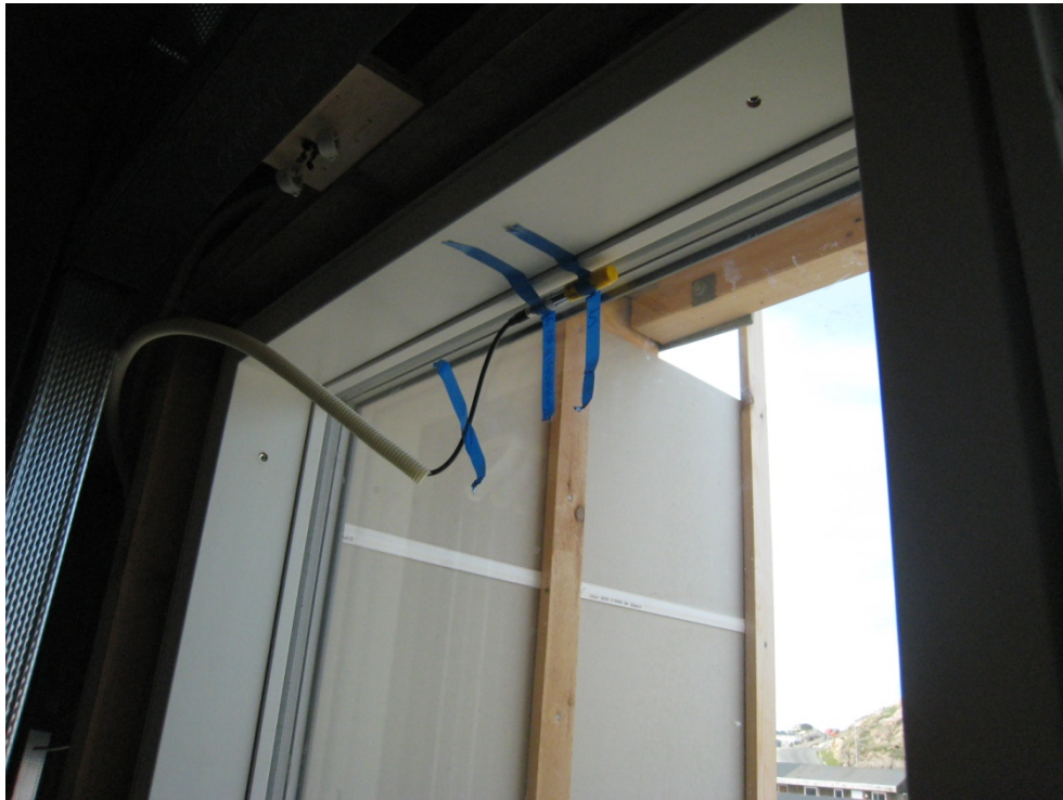
Fig. 24. Vaisala sensors, module line 3-4, DTU5 from inside, close-up
