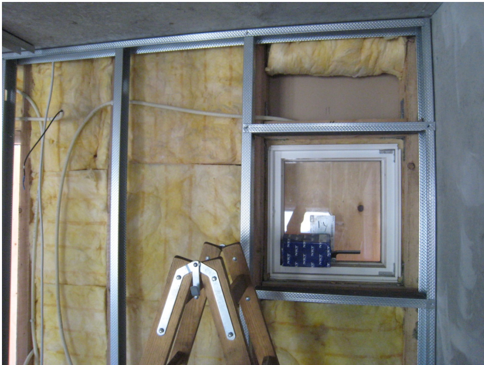
Fig. 34. Vaisala sensors, module line 3-4, DTU11 from inside
