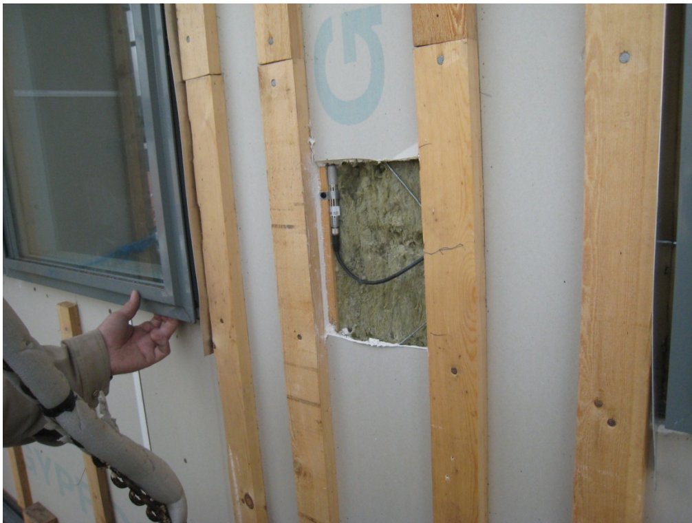
Fig. 18. Vaisala sensors, module line 3-4, DTU3 from outside
