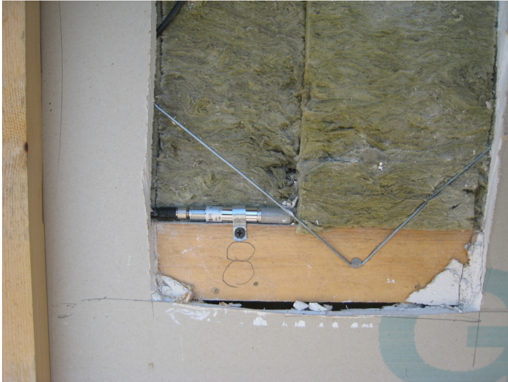
Fig. 29. Vaisala sensors, module line 3-4, DTU8 from outside, close-up
