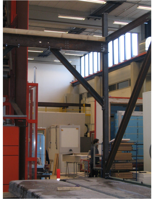
Figure 6.17 Pictures of the load bearing construction and the lower deck after installation.
