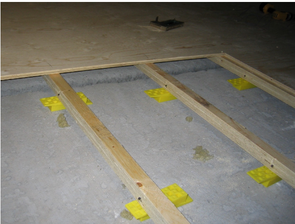
Figure 6.20 Floor construction. A wooden floor on rafts is used. A plywood plate of 15mm is used as the floor covering. In the room, a 6mm parquet floor is placed on top of the plywood plate.
