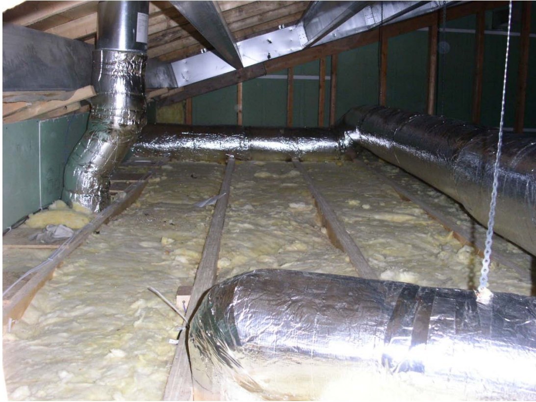
Insulated ducts in the cold attic.
