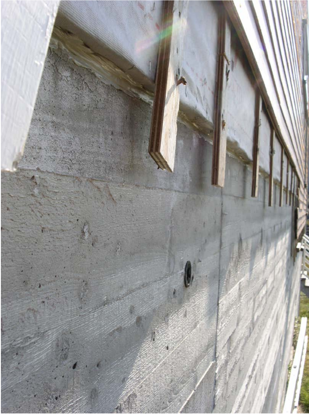
Improving the air tightness (summer 2010). The gap between wind barrier and wall has been sealed by silicon
