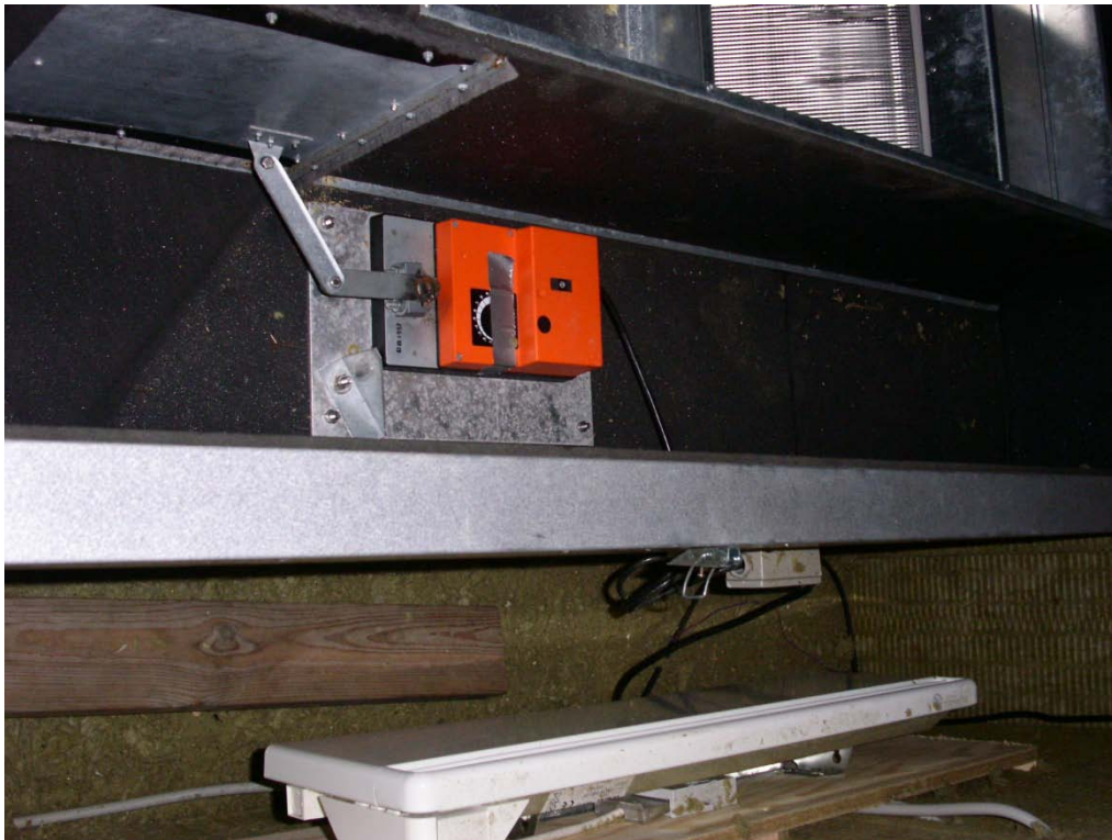
Mending the damper of the heat exchanger. The arm was welded to the servomotor.
