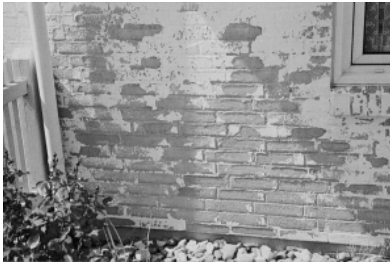
Figure 2.5 Peeling of coating from bricks which is mainly due to application of too large amounts of coating (Byggeskadefonden 1997)
