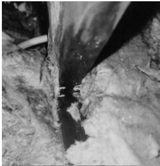
Figure 2.4 Example on decomposed wood components in a roof construction due to poor ventilation (Byggeskadefonden 1997)
