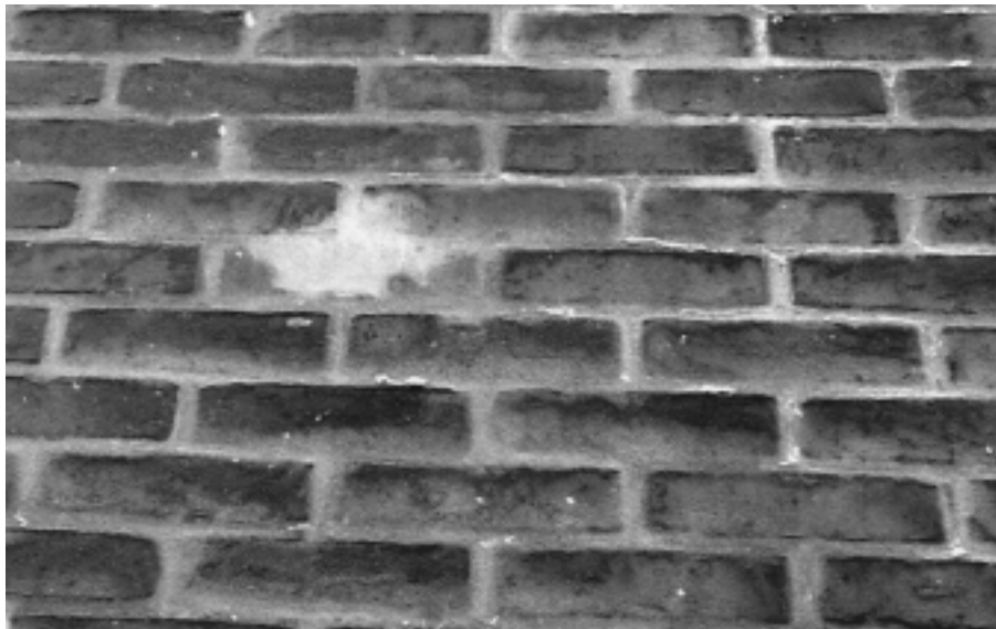
Figure 2.1 Example of salt deposits on brick wall surface following a wetting and drying cycle. The salt deposits are the small white spots at the picture in figure 2.1. The large white area in figure 2.1 is not a salt deposit but is due to a surface treatment during the experiment.
