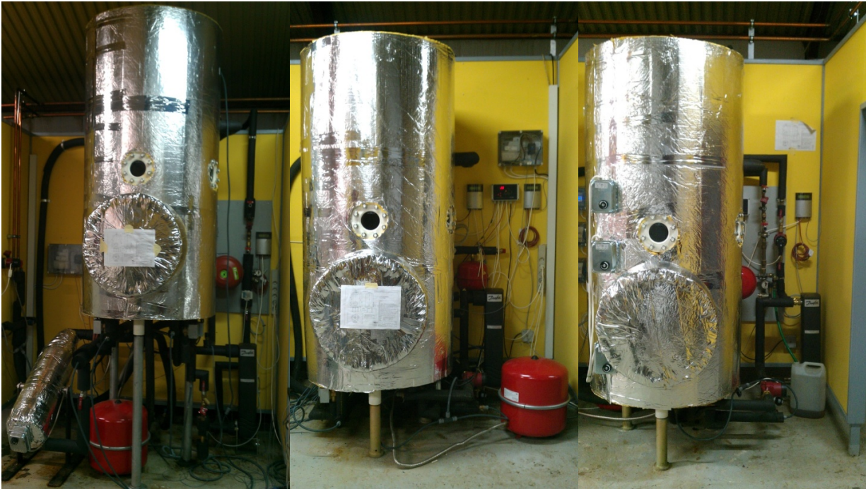
Figure 20. The heat storages of the three solar heating systems which are being tested.
