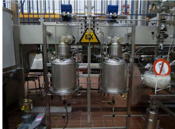
A pilot plant for enzymatic biodiesel production (reactor part)
