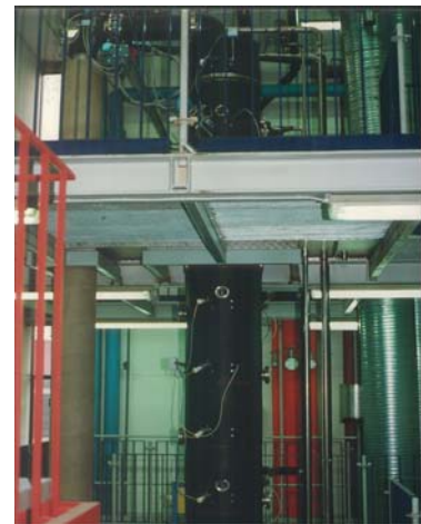
Indirect Vapour Recompression Distillation Pilot Plant
