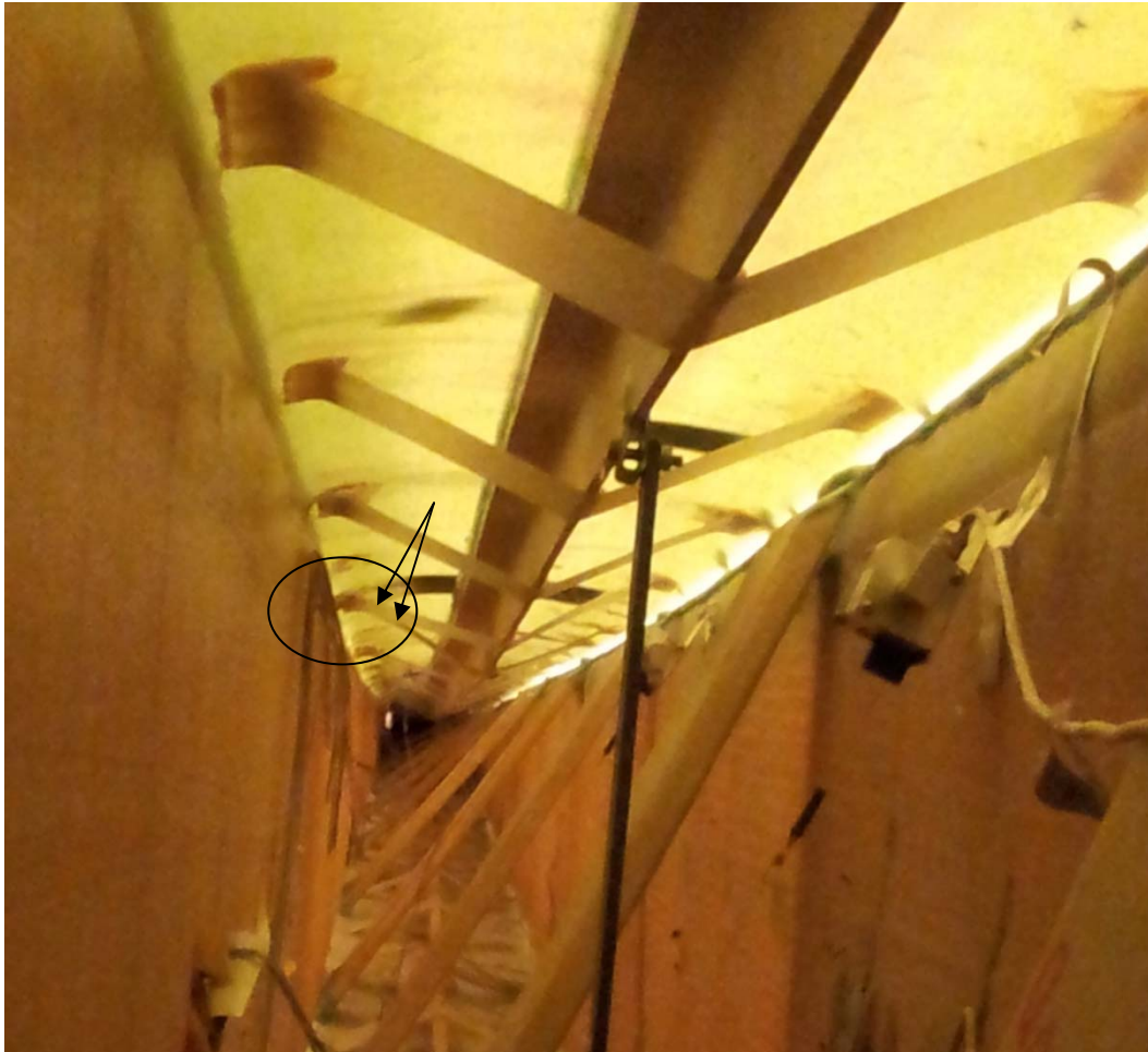
Figure 68 Photo inside the box after the test DMT_2012_05_31_A. the photo is taken inside the box, as it is difficult to get close to where the damage occurred. But examining it closely at the circle, one of the two transverse stiffener has debonded.
