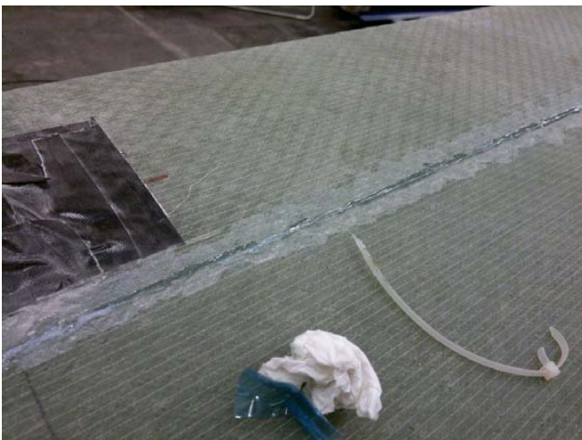
Figure 2. Close up on the bonded and smoothed out adhesive over the fibre
