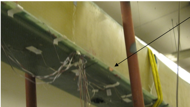
Figure 83 Steel pipe supporting the blade. There is a damage in the connection between the web and the cap
