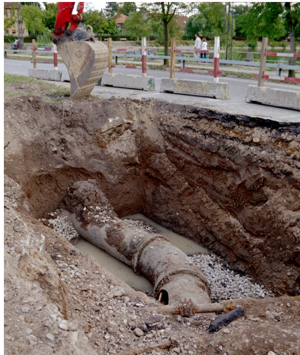
Figure 3-3. Burst pipe awaiting repair. Water is not properly drained from the hole. Photo: H.-J. Albrechtsen.
