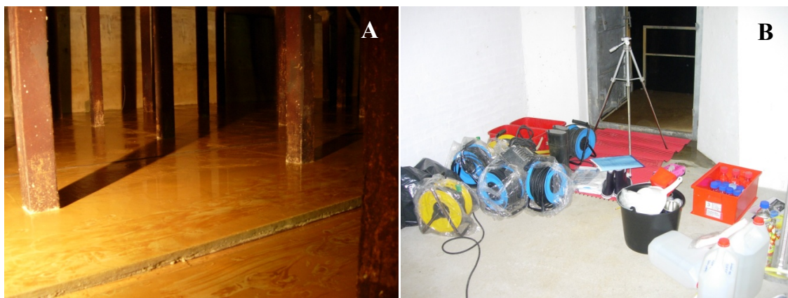
Figure 2-3. A) Empty clean water tank with reddish-brown sediment on the floor and a flush channel. B) Sampling equipment at the entrance of the tank. Photos: S.C.B. Christensen.
