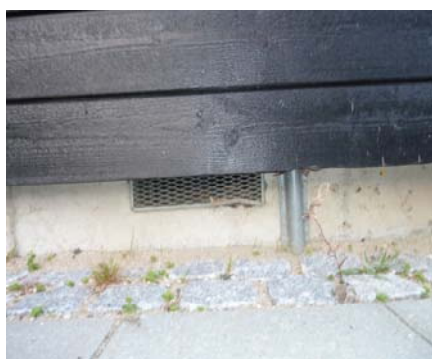
Figur 91 Ventilationsrist i fundament
