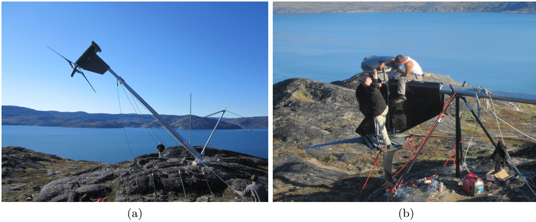
Figure 2.2: Work on the wind turbine at Sarfannguaq. (a) The turbine being put down - (b) Work on the brake pads inside the nacelle
