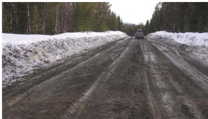
Figure 4-3 Frost damage on a gravel road in Raattama, Finland (photo J. Leskinen) [ www.tiehallinto.fi ]
