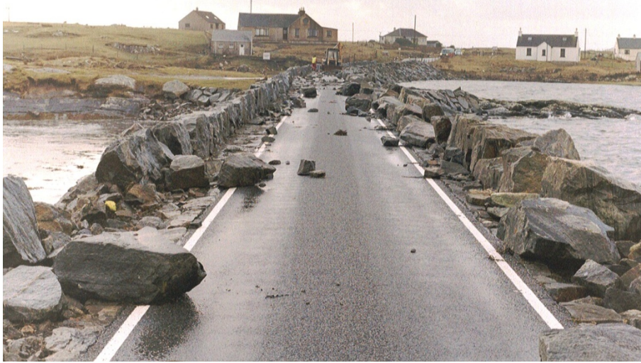
Figure 5-2 Damaged causeway in Scotland [ http://coastadapt.org/Outer-Isles/index.html ]
