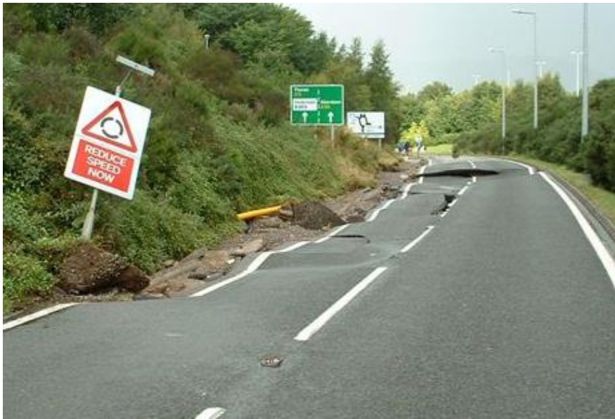
Figure 4-8 Damage to A9 Raigmore Slip Road, Inverness, 2002, following heavy rainfall. Photo by BEAR Scotland Ltd.
