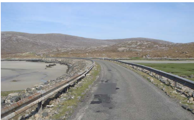
Figure 4-7 Lifeline coastal causeway on the Isle of Harris, The Western Isles, Scotland
