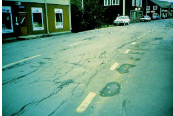
Figure 4-1 Frost heave on a city street in central Sweden. [ http://pavementinteractive.org/index.php?title=Frost_Action ]
