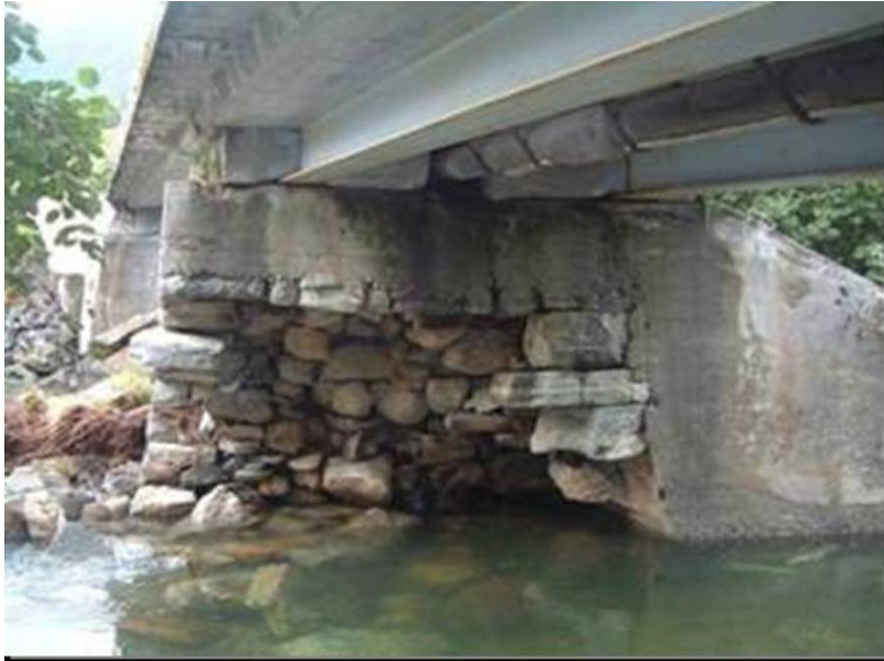
Figure 4-9 Bridge scour, Serkeland, Telemark, 2007 [photo from the Norwegian Public Roads Administration]
