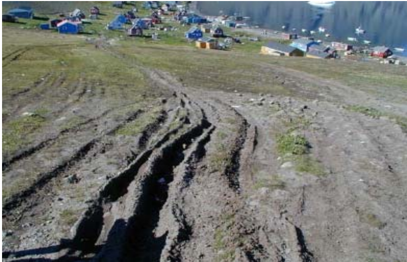
Figure 5-1 Rutting due to thawing of permafrost in Greenland
