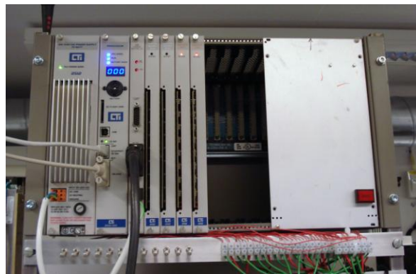
Fig 2: The new CTI system (In order from left: Power Supply, CPU, Interface card, 4 Analog 8 Channels IN/OUT cards)
