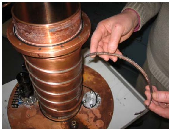
An attempt by BNL to replace burned fingerstock in situ failed. The cold solder joint held for a few weeks.
