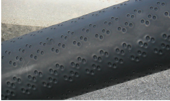
(a) Cable from the Tatara Bridge. Reproduced from Katsuchi and Yamada (2009b).
