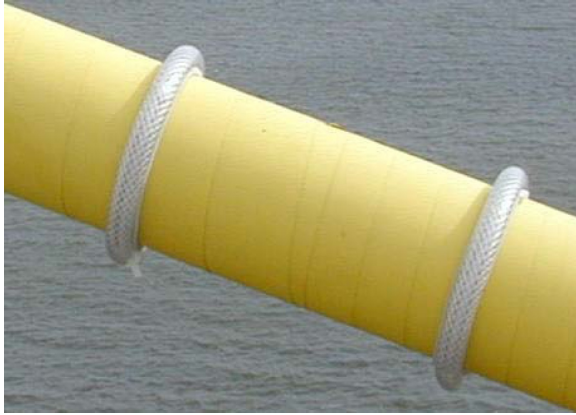
Figure 32: Circular rings mounted on two of the Veterans' Memorial Bridge cable-stays. Reproduced from Phelan et al. (2006) .
