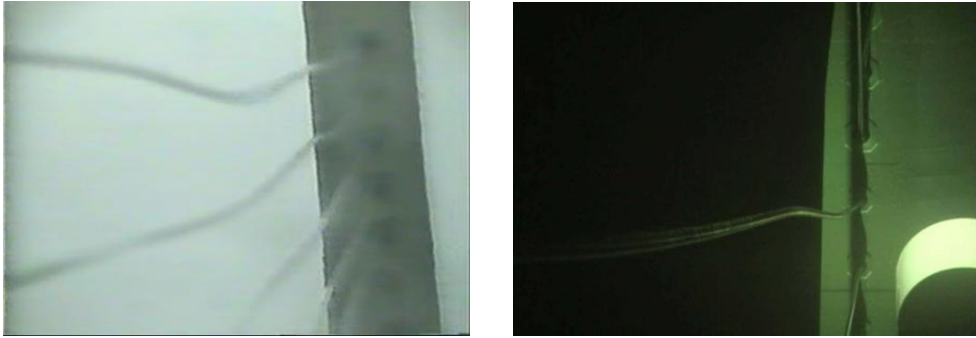
Figure 1.1: Photos of excessive cable vibrations. (left) is from Second Severn Crossing and (right) is from the Meikou bridge (photo by Prof. Tomomi Yagi ).
