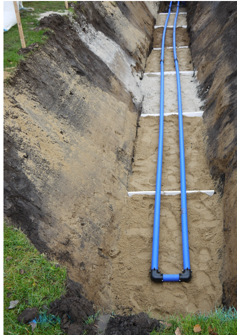
Figure C.1: Experimental setup under construction. Temperature and moisture content sensors were installed such that the moisture migration, caused by the hot water circulating the pipes, could be monitored.
