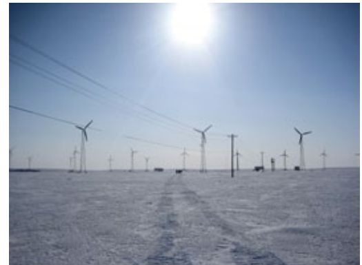
Kotzebue Wind Farm, Alaska 18
