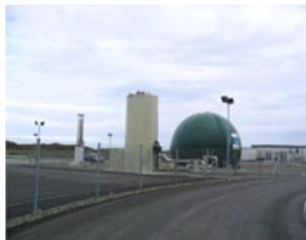
▲ The Biogas storage tank
