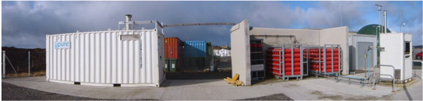
▲ Hydrogen production and storage systems
