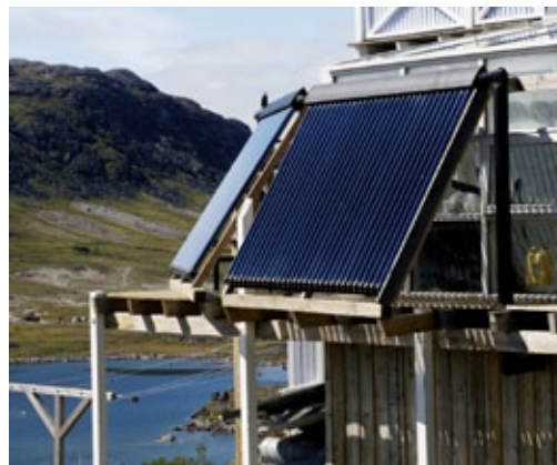
Solar Hot Water Panels, Qaqortoq, Greenland 13
