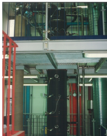
Indirect Vapour Recompression Distillation Pilot Plant
