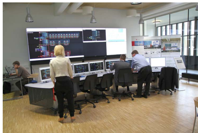
Figure 4. ControlLab + Scada system for education and research. The Scada system allows for monitoring and control of the main laboratory facilities including monitoring of the electrical power system on the island of Bornholm.
