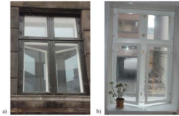
Fig. 4. Energy retrofitted 4-lite of type Window 2 with a secondary frame seen a) exterior of building and b) interior
