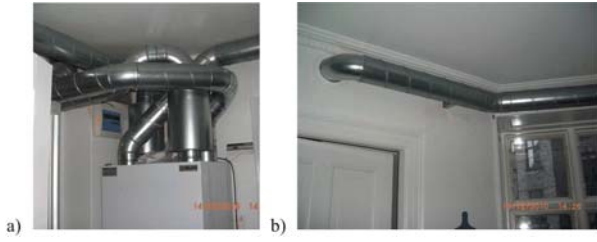
Fig. 10. Ventilation ducts in apartment. a) Inlet and outlet from the air handling unit; b) duct located in rooms
