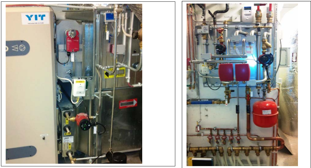
Figure 7. Close up of district heat supply heat exchanger in central air ventilation system (left), and district heat supply heat exchanger for DHW (right). Photos: The Author.
