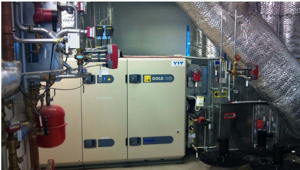
Figure 6. Forced air ventilation system with centrally placed rotating heat exchanger and subsequent district heat added as base load heat supply. Photo: The Author.
