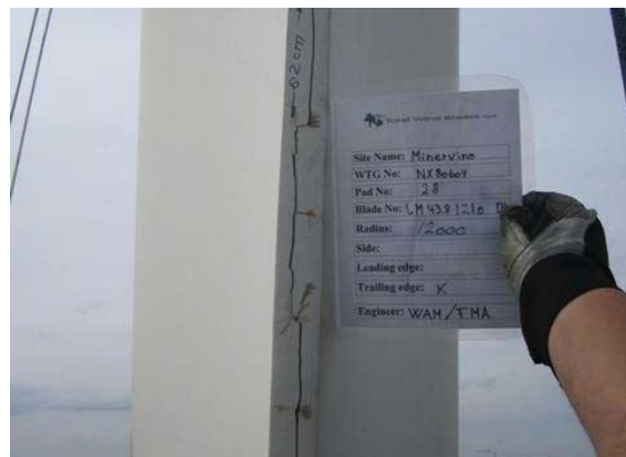
Figure 7 Fatigue failure in bondlines, longitudinal cracks in the trailing edge
