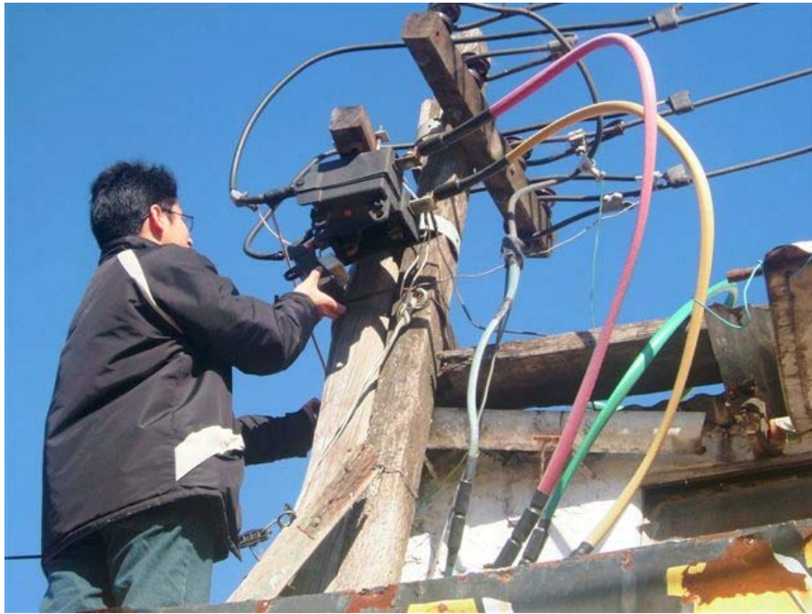
These connections are maintained by residents without any training, appropriate tools or protective clothing.
