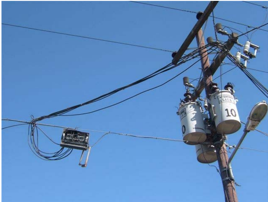
In many Barrios Carenciados (Type C), illegal 'hook-ups' are made to the grid where many, or most consumers have a formalised (metered) service with individual billing. The above photo shows how this is achieved through the tampering of overhead cables.
