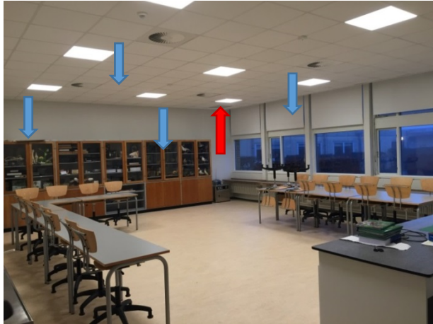
Fig. 3 Photo of classroom #2 with four swirl diffusers in the ceiling.
