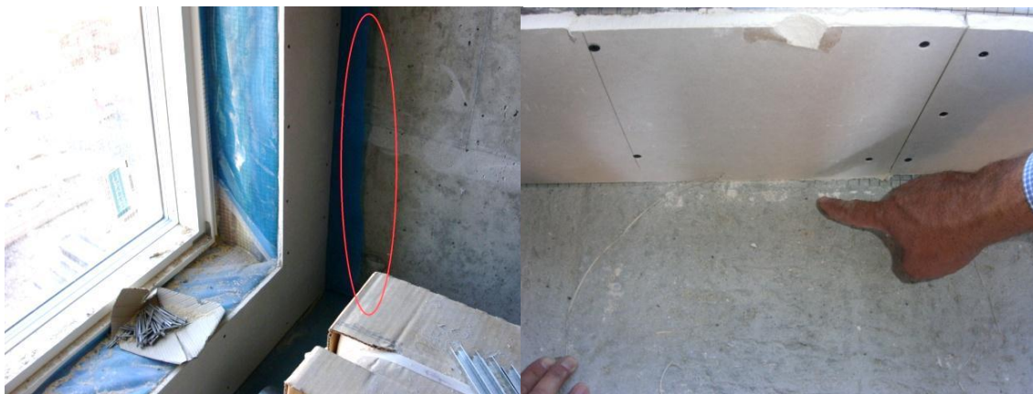
Figure 6. Left: Correct connection with overlap; Right: Missing overlap
