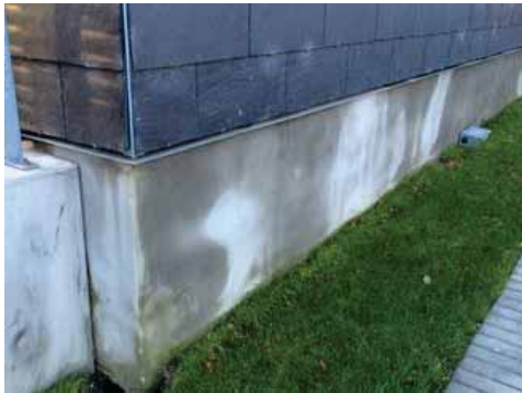
Figure 5: The water drops containing chloride ions run down the vertical MgO-boards and drain out of the wall from behind the wall's siding boards.
