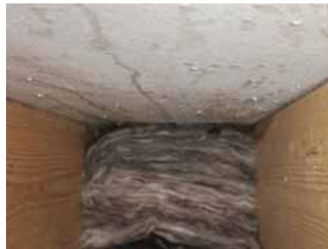
Figure 4: Salty water drops on a vertical MgO-board on the side that faces the insulation filled cavity inside the wall.
