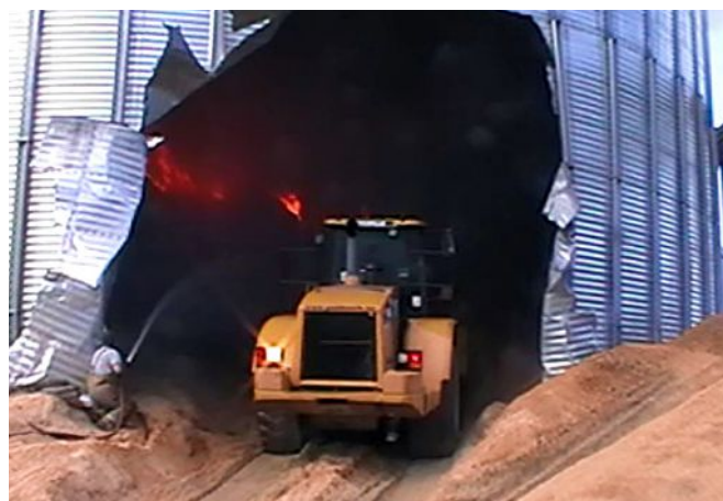
Top: Water is often an unsuccessful method of fighting smouldering fires in bulk storage silos.
