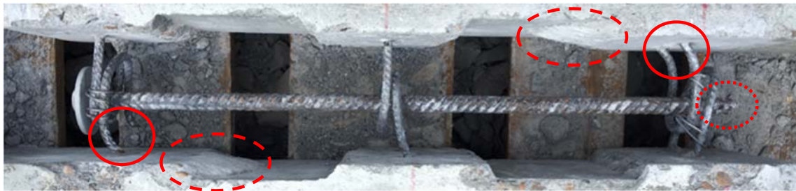
Figure 5. Example of post-test observations of extensive U-bar deformation (red circles), rupture of locking bar (red dotted circle), and local mortar failure in the key corners (red dashed circles), Specimen C3.
