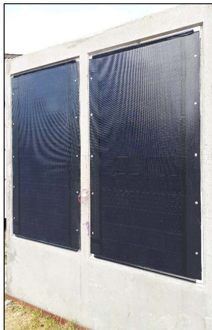
Fig. 1: PVT collectors integrated into a concrete facade.
