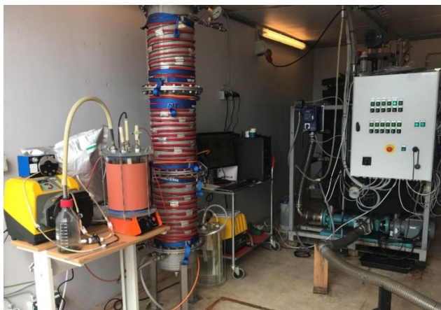
Fig. 5. Pilot-scale operation at BIOFOS WWTP in Avedøre
