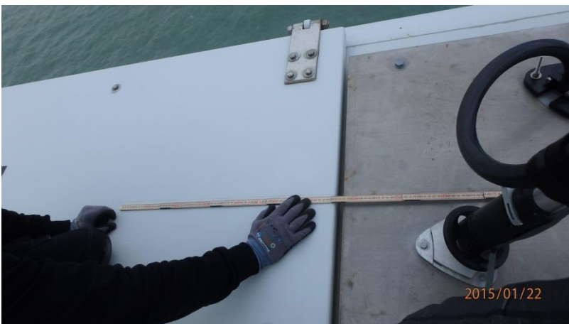
Figure 20 Alignment of the Wind Iris optical head (using the red leads – one in the back, shown on the picture, and one in the front, not shown on this picture) to the turbine shaft (represented by a line drawn on the nacelle roof).
