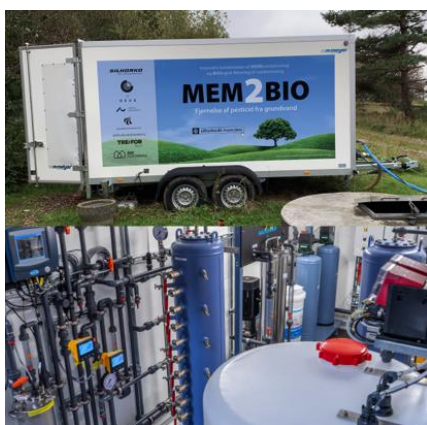
Figure 1: Pilot plant at the site in Esbjerg
