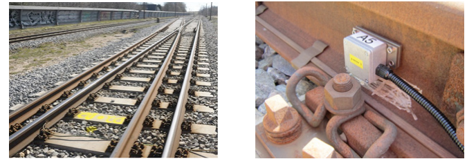
(a) Overview of the turnout close to Tommerup station.
