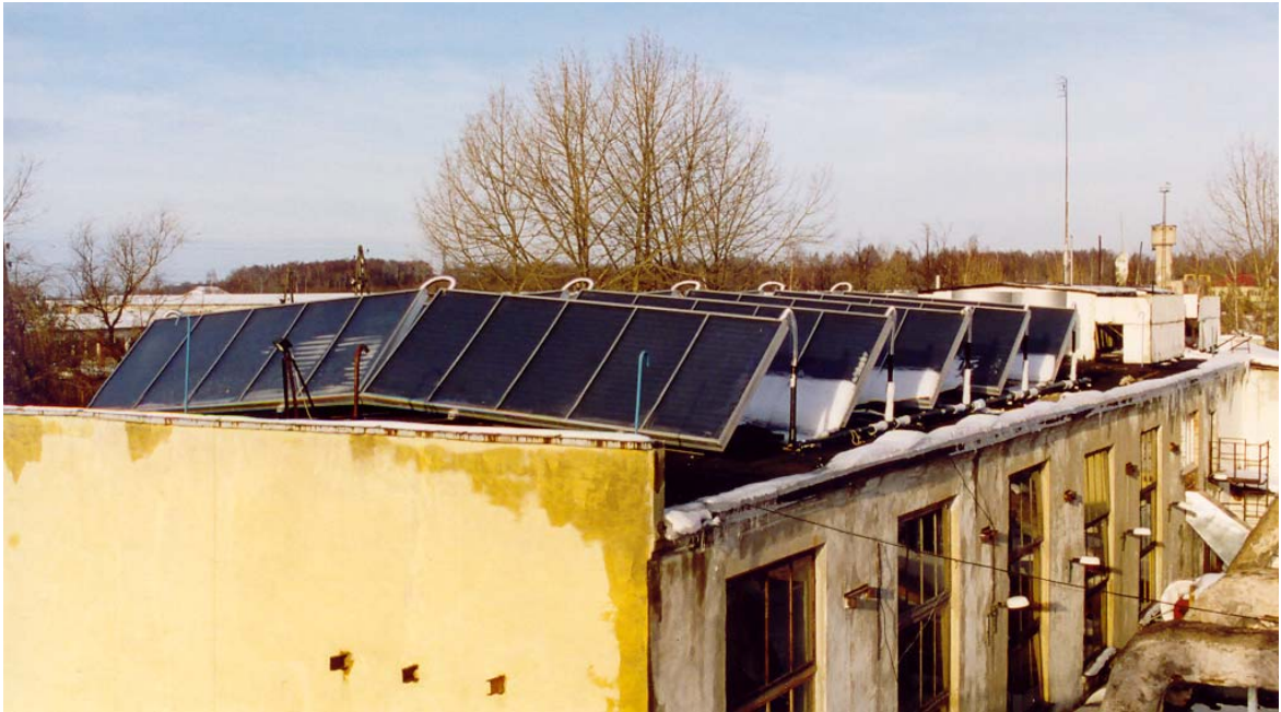
Fig. 9. Photo of the solar heating plant.
