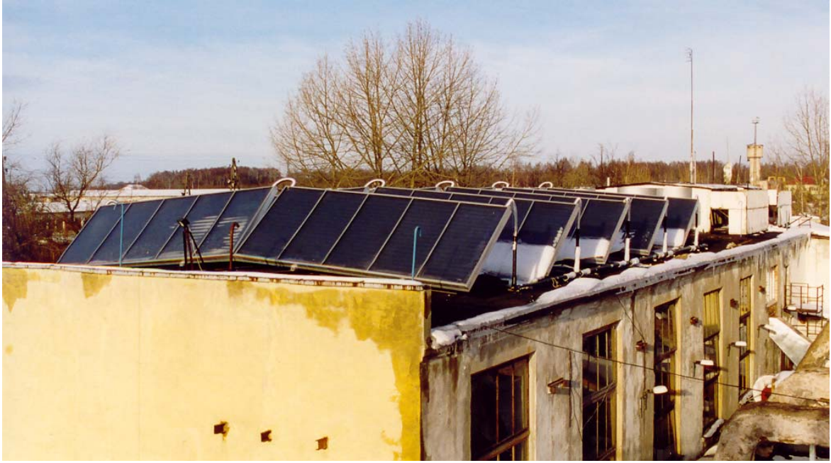
Fig. 9. Photo of the solar heating plant.
