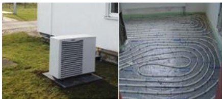
Figure 3: Heat pump and the underfloor heating system
