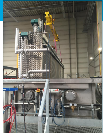
Cold store evaporator, 7 meters long, 160 kW cooling capacity
