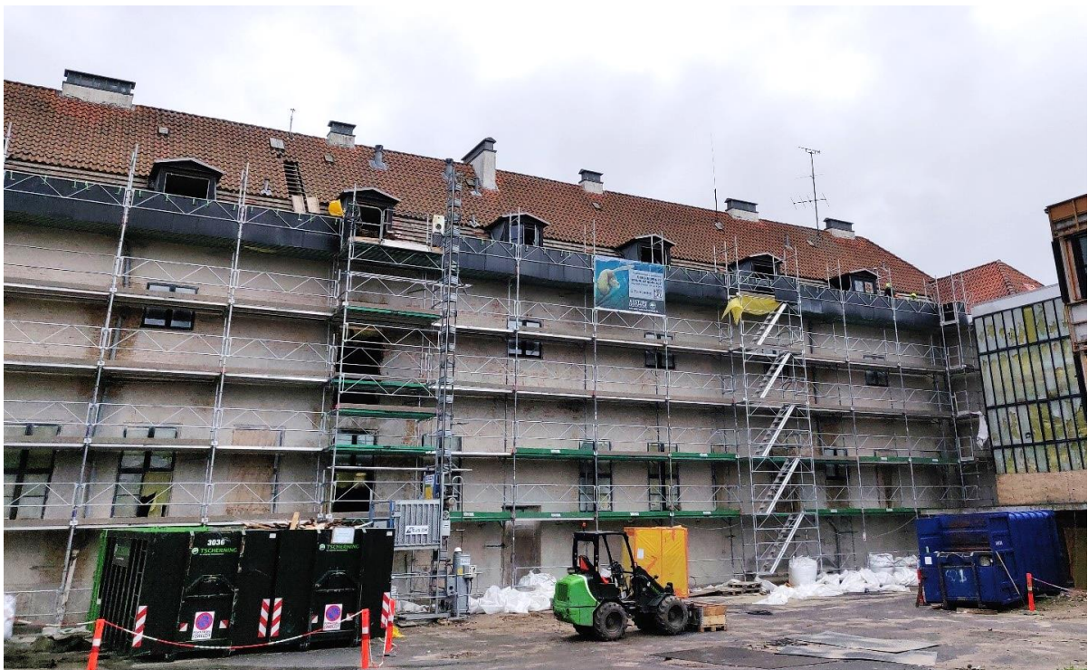
Figure 20. Selective demolition of roof tiles using scaffolding (photo provided by Tim Riis Tolman, Lendager TCW).
