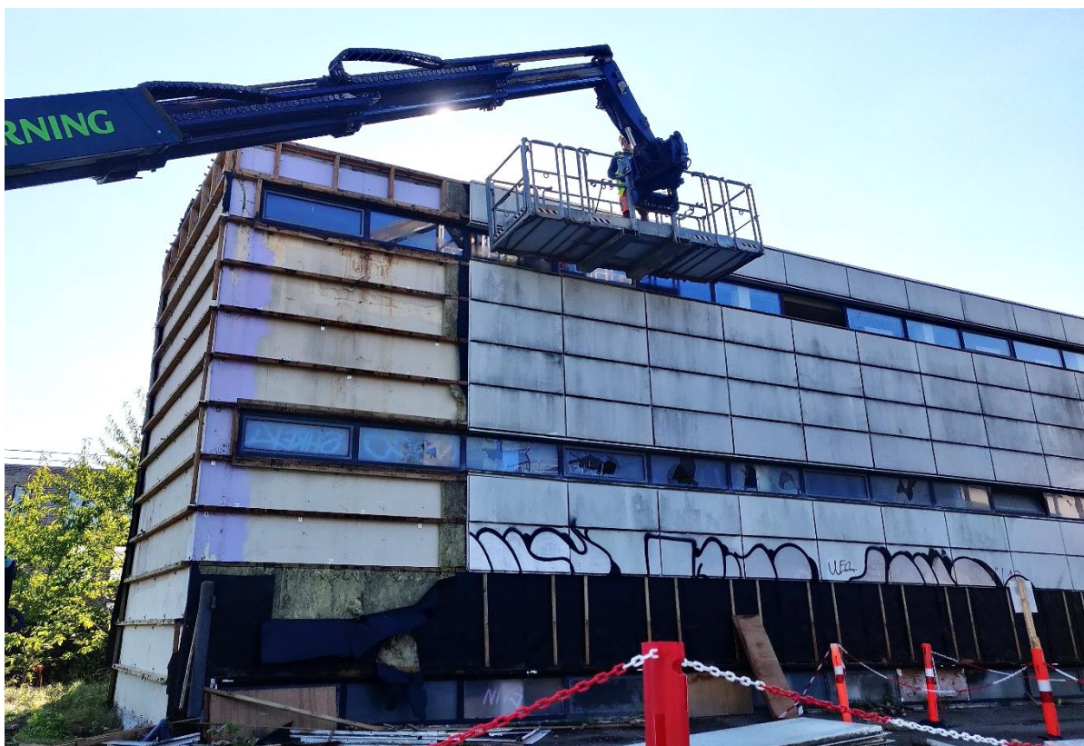
Figure 21. Selective demolition of façade cladding using a mechanical lift (Photo provided by Tim Riis Tolman, Lendager TCW).
