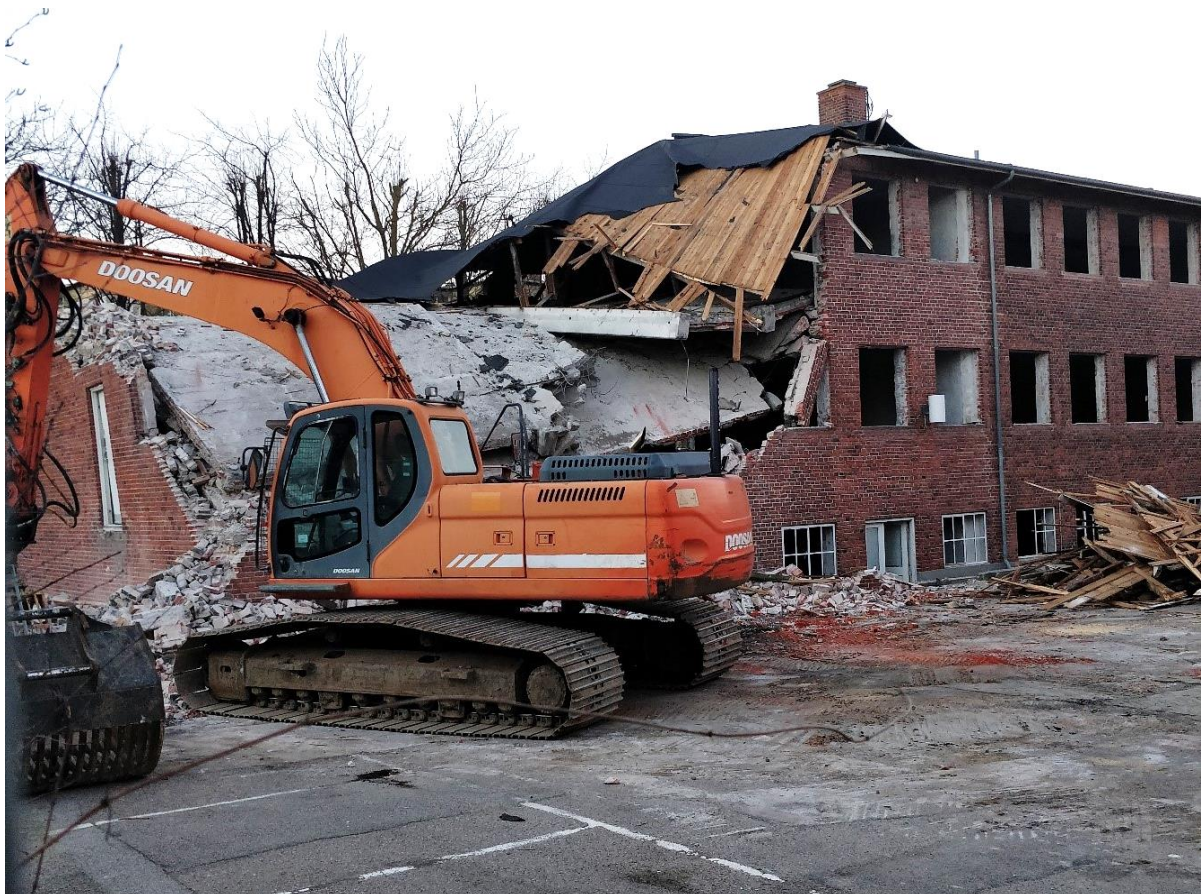
Figure 19. Conventional demolition of office building. The windows and fixtures have been removed in advance, but the remaining building parts will be demolished and sorted on site.
