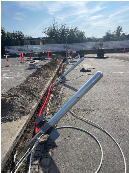
Figure 8: Cables are in the ground and poles are ready to be fixed in the ground.
