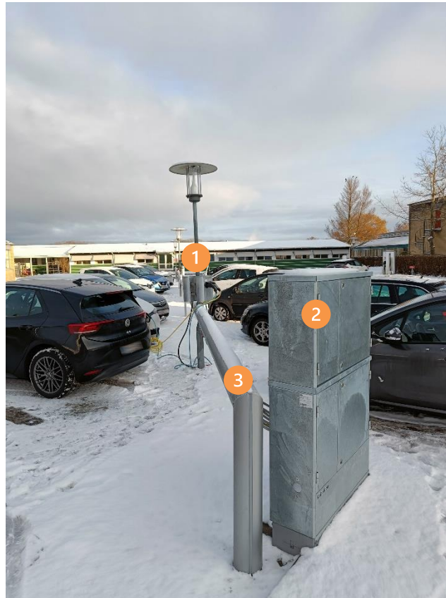
Figure 2: Charging infrastructure in Risø. 1) Chargers; 2) PCC cabinet for all EVSE connections; 3) Cable tube for connecting chargers to PCC cabinet.
