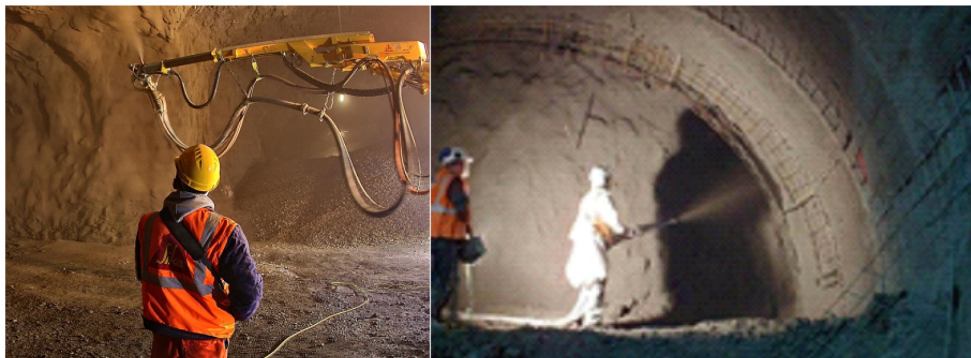
Figure 1. Example of current shotcrete activities. (Images taken by authors during relevant construction activities).
