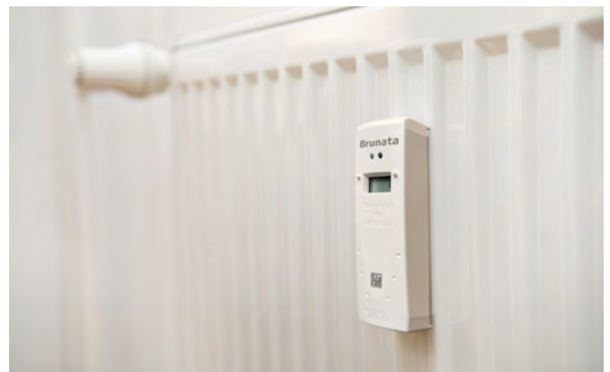
Figure 2: Typical radiator in apartment buildings with thermostatic control valve and heat cost allocator
