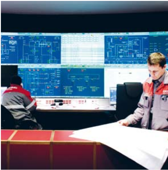
Source: Dong Energy
