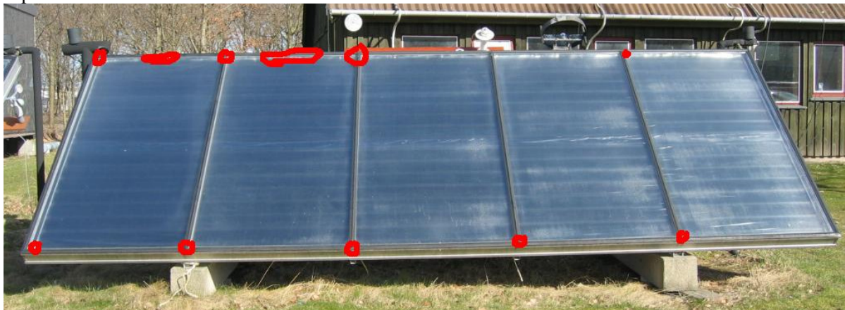
Figure 13. Damage of the Teflon layer in the collector from Marstal.
