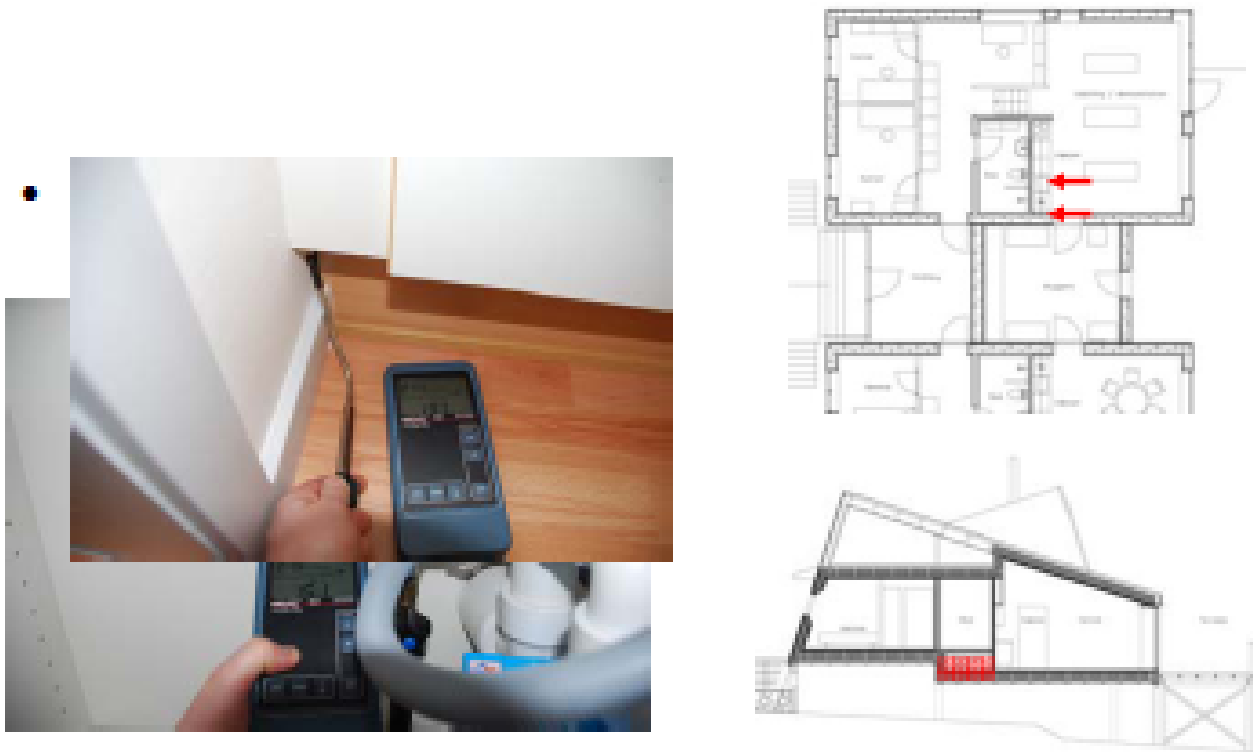
Figure 28 Leakage between kitchen unit and crawl space (shaft)
