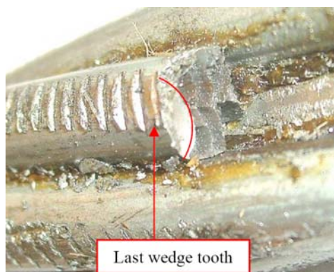
Fig. 4 Wire fracture at simple anchorage
