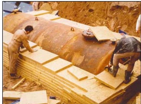
The enormous heat storage tank.
