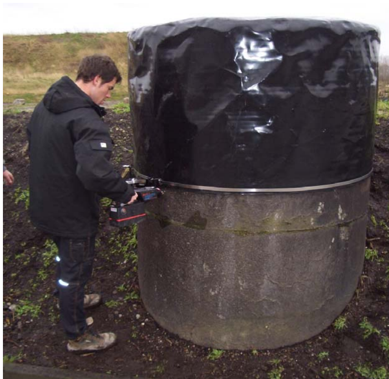
Figure 3. Leachate well gas barrier installed on a leachate collection well at Fakse landfill
