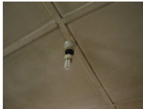
Insulated ceiling and CFL lamp installed in one of the demonstration houses.
